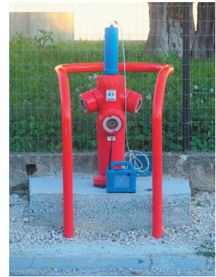
Fire hydrant injection
